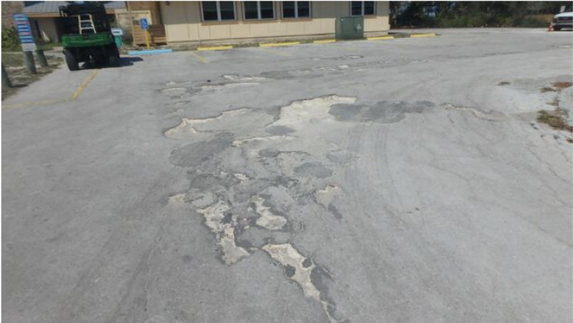
Figure 1. Parking Lot Existing Condition
